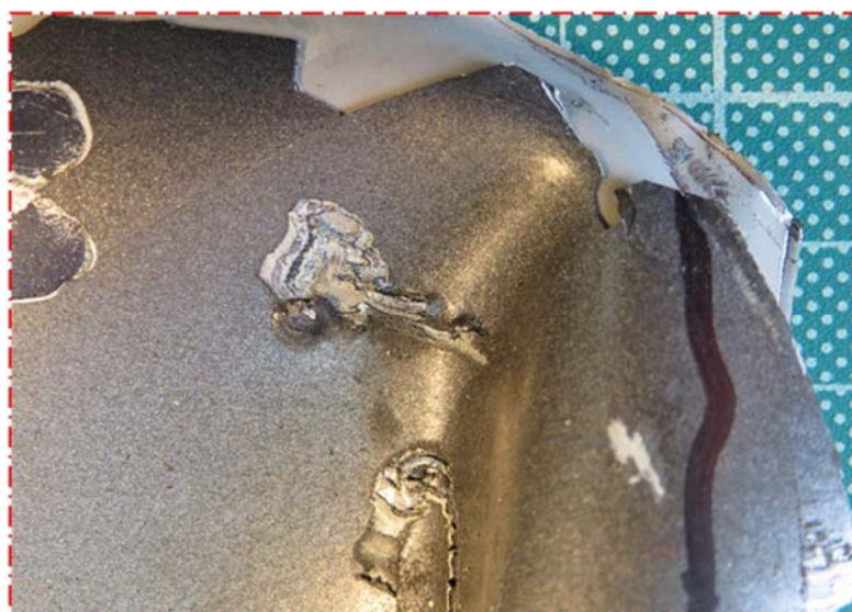
Photo 28: Detail B, the characteristic traces of the electric arc that was created between the metal cover and the Power Cables.
