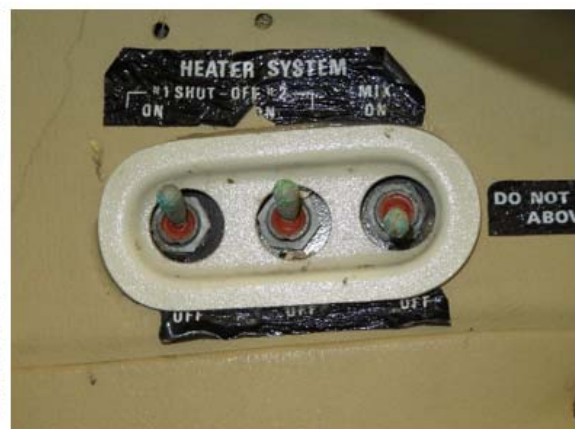
Photo 49: The cabin heating system switches.
