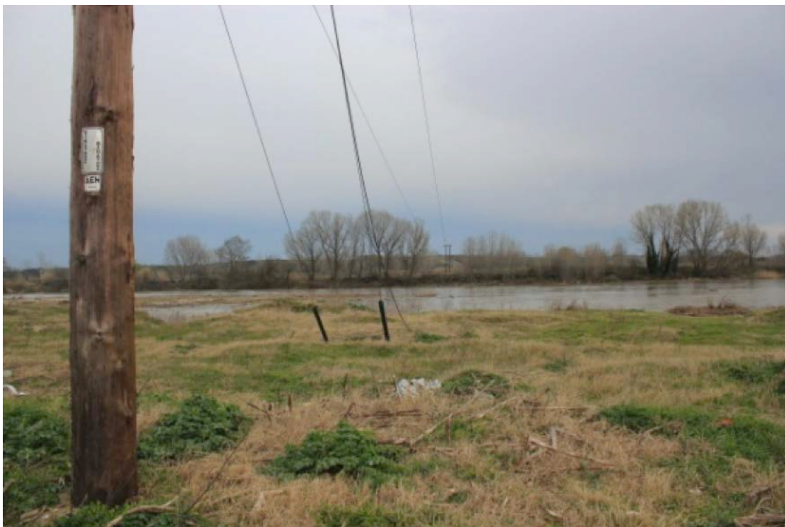
Photo 6. Public Power Corporation pylons, the damaged cables and the severed cable
